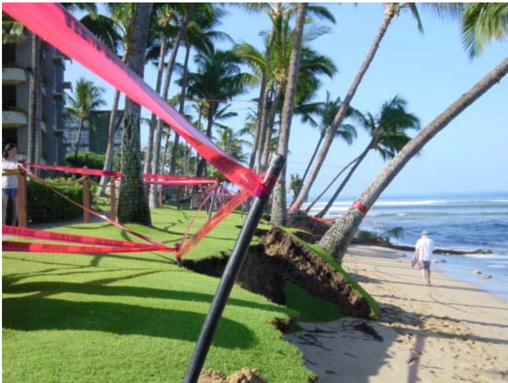
Figure 2 - Erosion event July 2003 at Hanakao'o Point.
