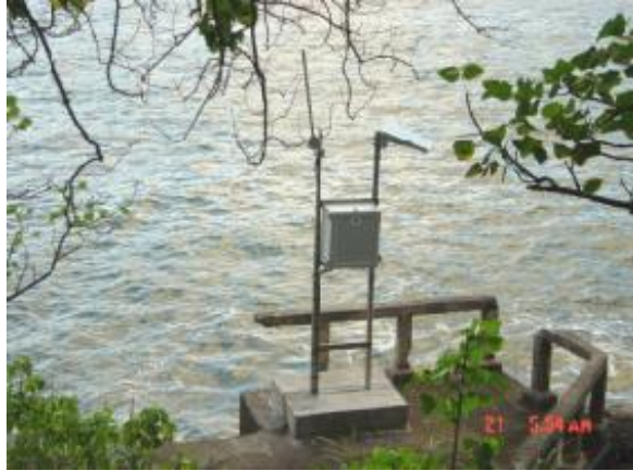
Hiva Oa Installation
