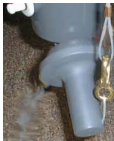
Incorrect - connection on side of bottom end cap
