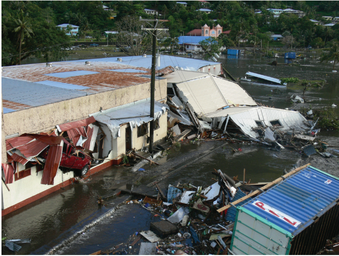
Figure 4 The 2009 tsunami in Pago Pago Harbor, American Samoa. This image shows water draining off the land after the tsunami did extensive damage to the community.
