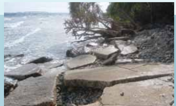
Erosion on atoll islets has undermined and damaged infrastructure built during WWII. (Source: C. Fletcher)
