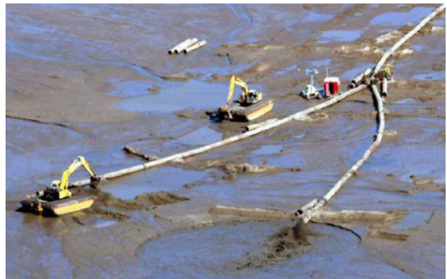
Sediment dredged from navigation and diversion channels can be used to restore and create wetlands.
