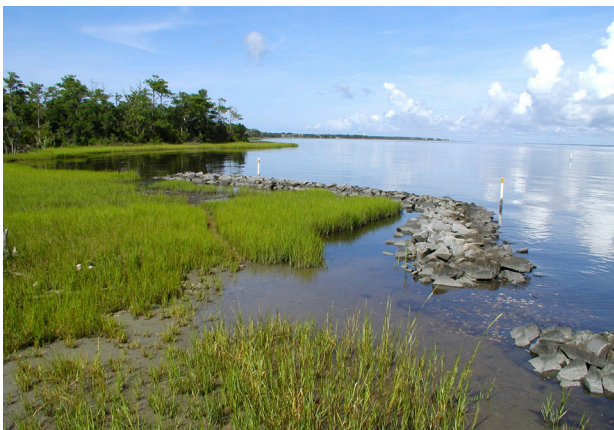
Hybrid shoreline stabilization structures that employ marsh plantings and low rock sills (to protect the vegetation) can help stabilize eroding banks.
